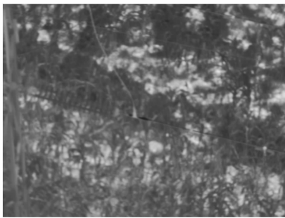
图15 发热极弱、背景复杂导致引流子故障不明显 Fig.15 Drainage fault is not obvious due to the very weak heat and the complicated background
